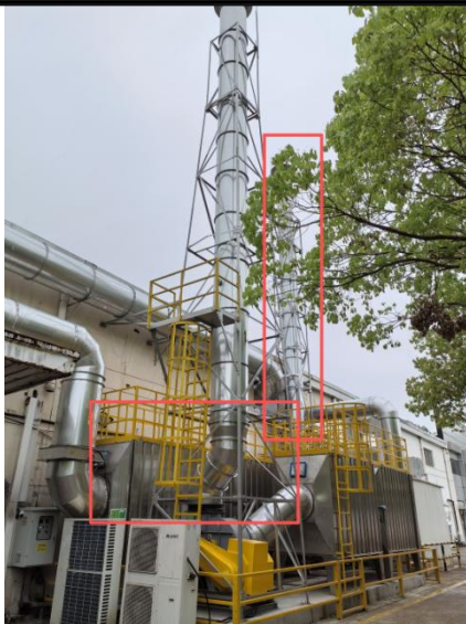
“初效过滤+二级活性炭”及 DA001 排气筒
