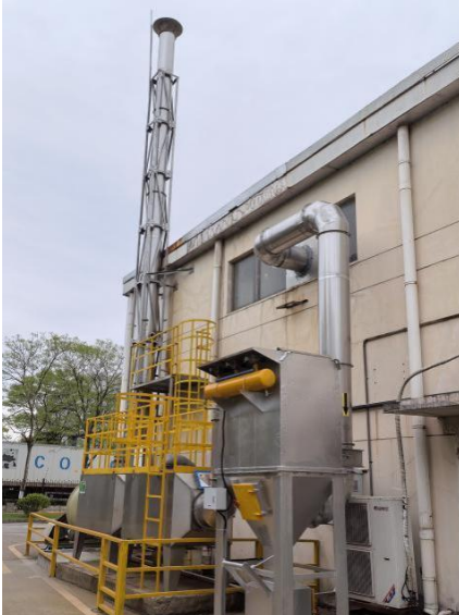
“滤筒除尘器+二级活性炭”及 DA005
