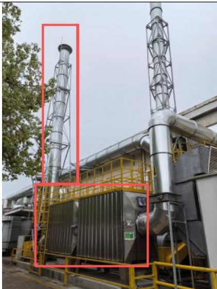
“初效过滤+二级活性炭”及 DA003 排气筒
