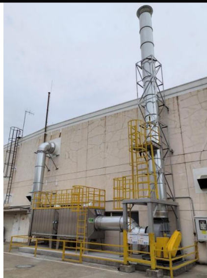
“初效过滤+二级活性炭”及 DA002 排气筒
